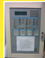
Fire alarm & evacuation systems
